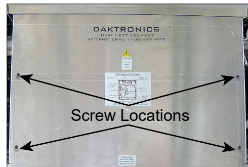
Figure 29: Control Equipment Door
