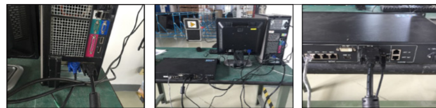
Figure 25: Connection from Computer (Left) to Rear of Sending Box (Right)
