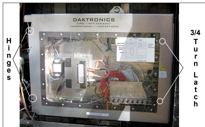
Figure 34: ISP Enclosure Cover Removal
