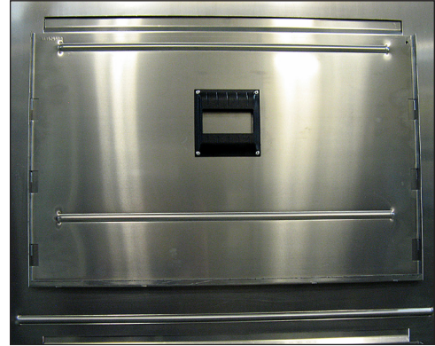
Figure 36: Control Equipment Door
