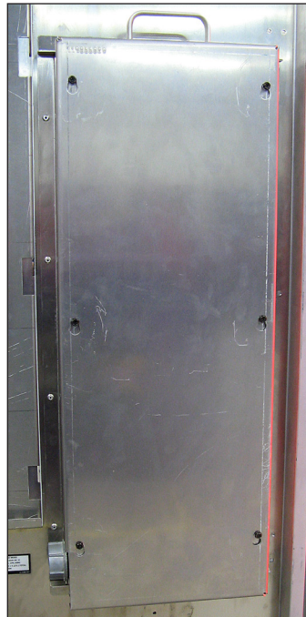
Figure 27: Power Entrance Access
