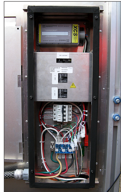
Figure 28: Power Entrance Box
