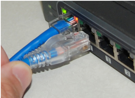
Figure 31: Network Hub Connection (2)
