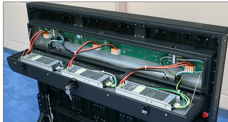
Figure 46: Power Supplies in Power Box
